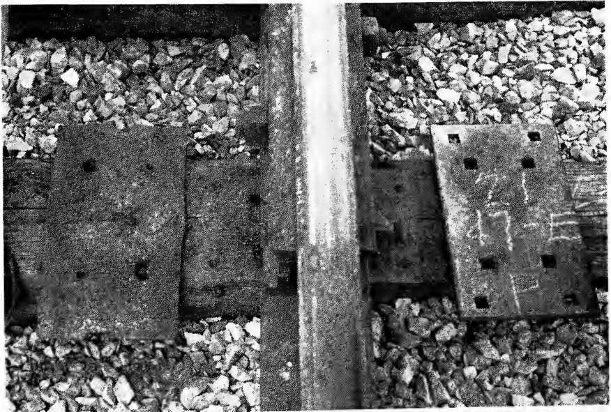
Fig. 25. Section 21, 13-in Fabco Tie Pad, Uncoated, After 83-months' Service on a Creosoted Pine Joint Tie in Tangent Track
